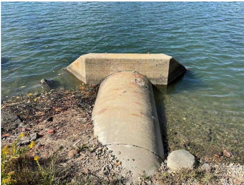
Photo 2 – Existing outfall headwall and exposed 48” RCP pipe looking northwest at approximate high tide. Taken 9/28/22
