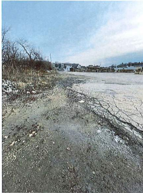
Photo 5 – Edge of concrete block wall at 90 Maplewood Ave LLC lot (right) looking northeast over existing pipe. Taken 1/19/23
