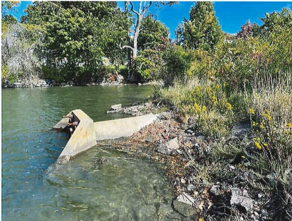
Photo 2 – Existing outfall headwall, exposed 48” RCP pipe, and tidal embankment looking east at high tide. Taken 9/28/22
