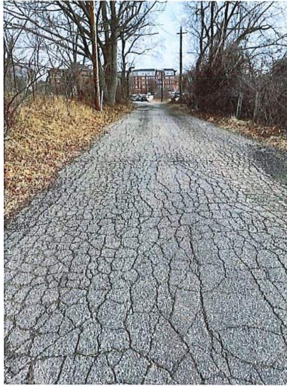
Photo 7 – Road between railroad (right) and Old North Cemetery (left) looking northeast toward Maplewood Ave. Taken 1/19/23
