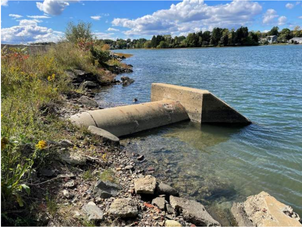
Photo 1 – Existing outfall headwall, exposed 48” RCP pipe, and tidal embankment looking west at approximate high tide. Taken 9/28/22
