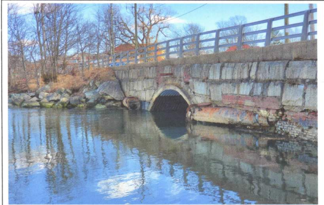
FIGURE 1 Arch Culvert at Maplewood Avenue Over North Mill Pond, Portsmouth, View Southwest of Seaward Side of Culvert from Shoreline (2/28/2020)
